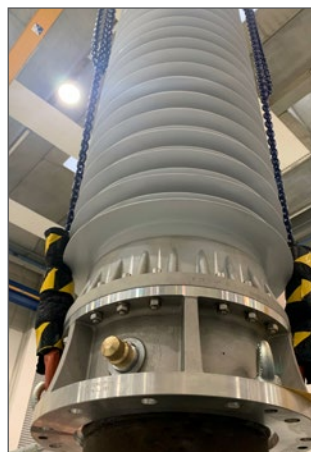
Fig.7/8: Lifting of the Bushings
