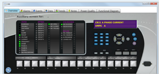
Tab Displays provide centralized, consistent control interfaces for substation equipment and IEDs
