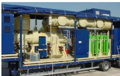
GAS NATURAL FENOSA (SPAIN) 132/66 kV 4 GIS bays
