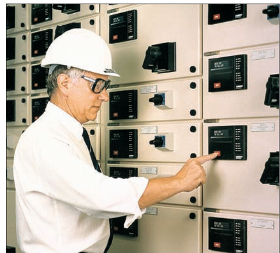
One MM2 is typically mounted in each starter of a motor control center.
