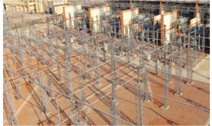
Typical AIS installation
