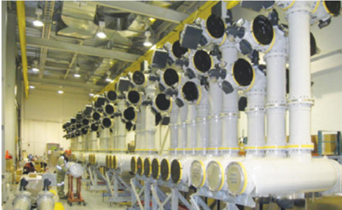
Typical GIS installation
