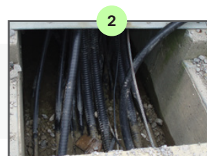
Traditional cable trenches
