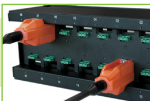
Fiber cross connect panels replace copper terminations
