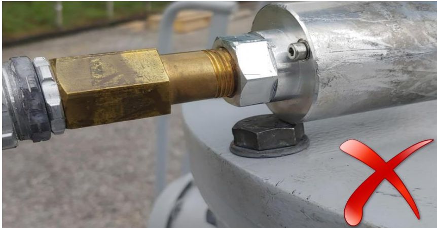
Figure 11-13: Bushing adaptor installation – bad / aborted example #1
