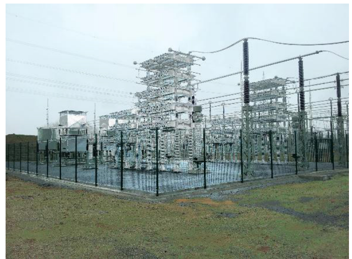
MSCDN installed in Germany
