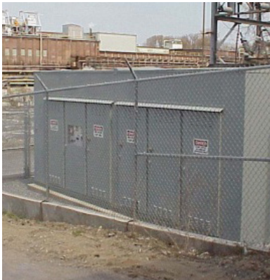
Metal Enclosed Shunt or Filter Bank
