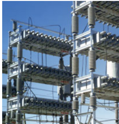
Open Rack Harmonic Filter Bank
