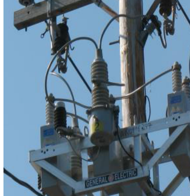
Pole Top Shunt Banks
