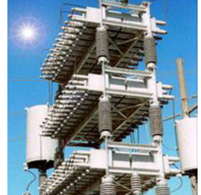
Open Rack Shunt Banks
