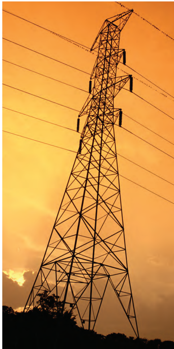
Figure 1. Overhead transmission lines
