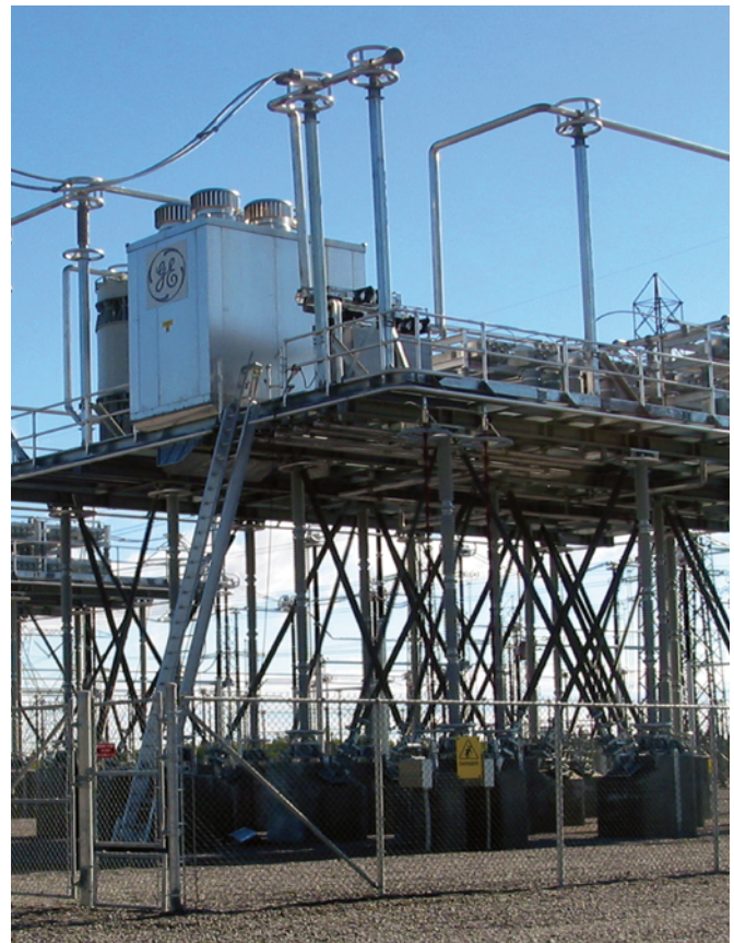
Figure 1. Photo of a series capacitor installation.
