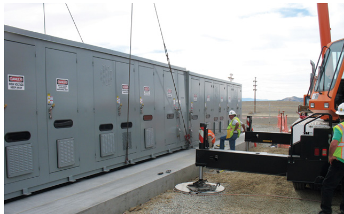
60 MVAR, 38kV, 5-stage 2 section Metal-Enclosed Capacitor Bank being installed at solar plant
