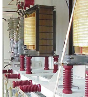
Iron-core harmonic filter reactors used in a 7 MVAR 5th harmonic filter bank. Note extensive use of plated bus for connection of reactors to capacitors.
