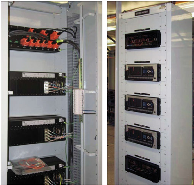
Figure 2. HardFiber protection panel with three relays and two patch panels (top and bottom). All I/O signals interfaced via fiber optic communications.
