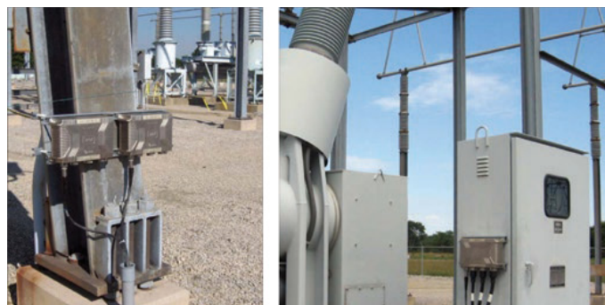
Figure 4. HardFiber bricks installed on a bus support structure (left) and a breaker marshalling box (right).
